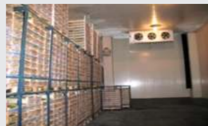
Chilling Chamber at Peca Komerc Supported by AgBiz
